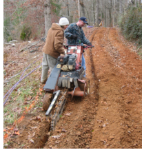
Sometimes you have to pump effluent to the top of a big hill.
